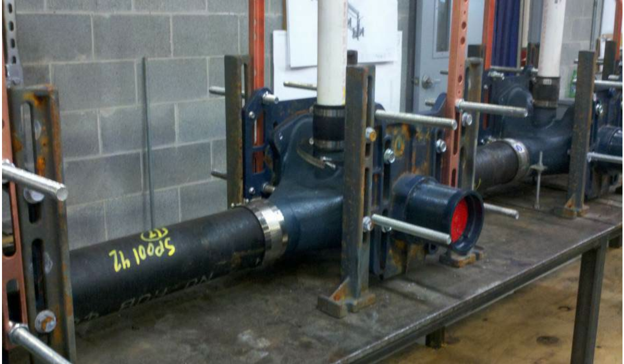
Shop fabricated pipe and wall hanger pipe spool
